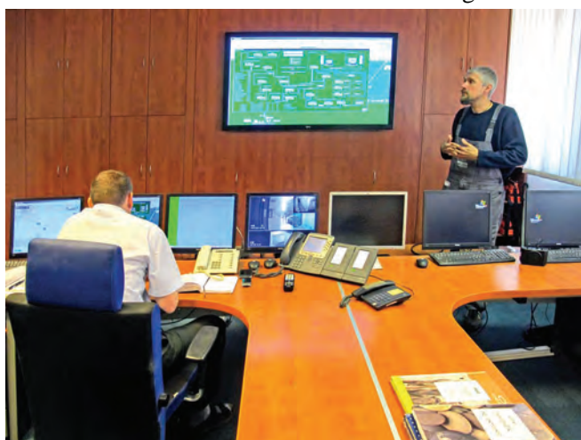
The Kolektory Control Centre with screens monitoring everything from temperatures and pressures to CCTV images
